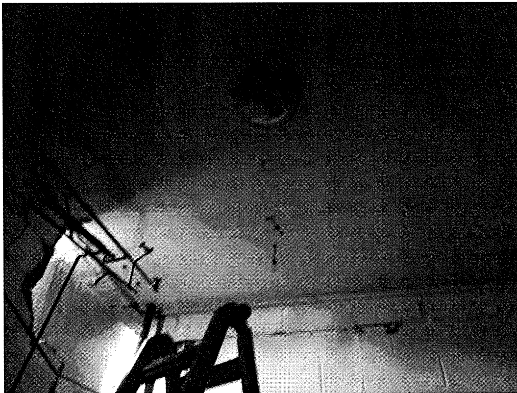
Ground Level: Asbestos containing ceiling joint compound and contaminated by layering ceiling gypsum.
