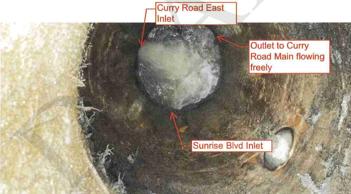
Manhole 54 A – Curry Road Tie in adequate capacity. Significant flow from Curry Road East. Our inlet on the bottom of the picture outlet on the top.
