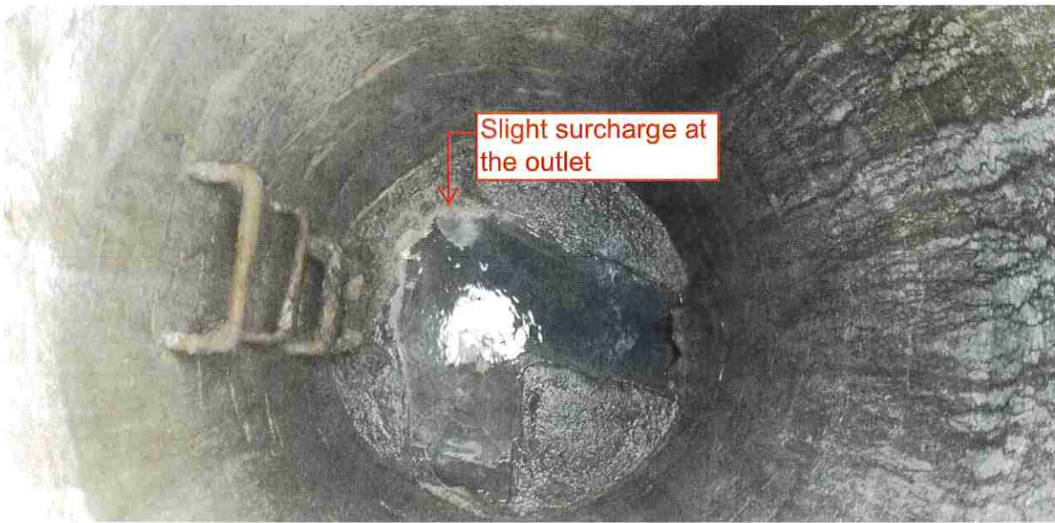
Manhole 314 A – Inlet out surcharging
