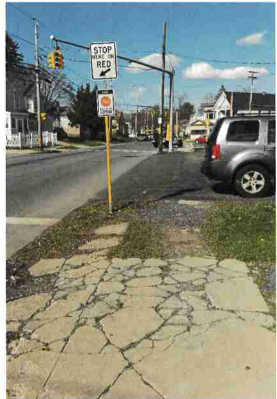
Figure 8: Sidewalk crumbling near Guilderland Ave/Genesee St
