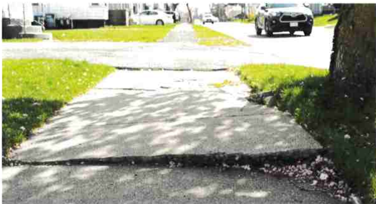
Figure 7: Sidewalk upheaval near Guilderland Ave/Genesee St
