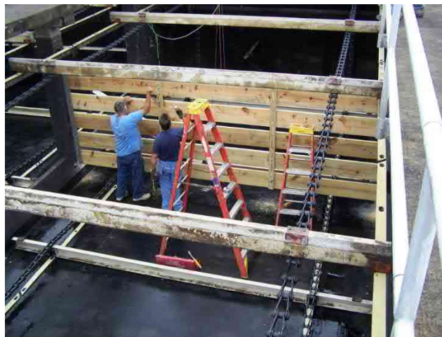
Figure 5-1: Typical Clarifier Baffle Installation
