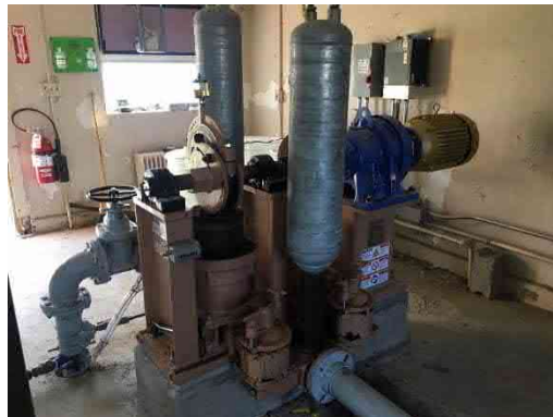
Figure 3-9: Belt Press Feed Pump
