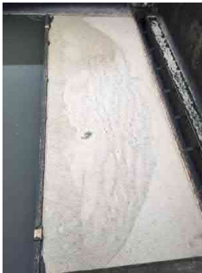
Figure 3-5: Primary Clarifier Grease
